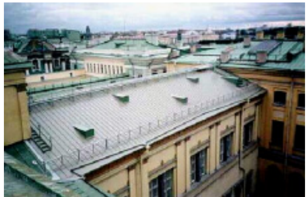
Hermitage Museum, St. Petersburg, Russia Gerard Prins, Architect Evers Partners, Consulting Engrs
