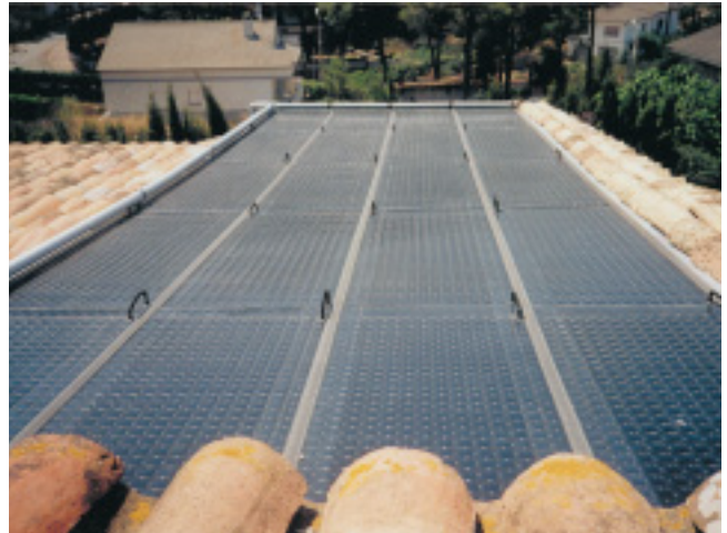
Casa Lledoner in Vallirana (Barcelona, Spain) (Photo: Energie Solaire Hispano Swiss SA)
