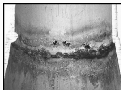
Corrosion damage in poorly welded joint | 15 mm grade X6CrNiMoTi 17-12-2/1.4571
